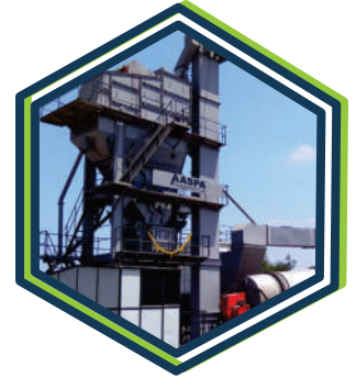
ASPHALT BATCH MIX PLANT
