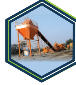
WET MIX DLC PLANT
