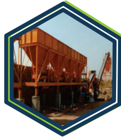
WET MIX MACADAM PLANT
