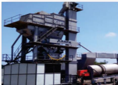
ASPHALT BATCH MIX PLANT
