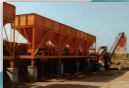
WET MIX MACADAM PLANT/DLC PLANT
