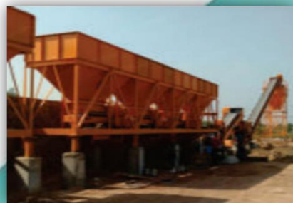
WET MIX MACADAM PLANT/DLC PLANT
