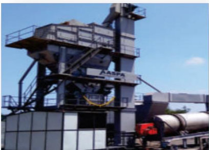
ASPHALT BATCH MIX PLANT
