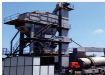
ASPHALT BATCH MIX PLANT
