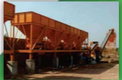
WET MIX MACADAM PLANT/DLC PLANT
