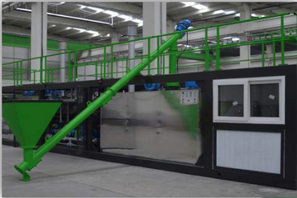
BITUMEN EMULSION PLANT
